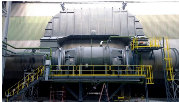
Figure 5. An EHEX type heat exchanger installed in line 4 at Aluminium Bahrain (Source: REEL Norway).
